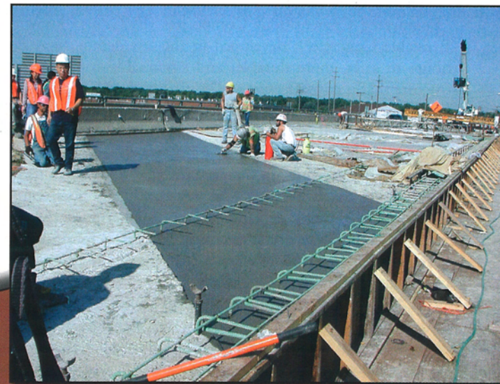
Figure 3a: Completed ECC Link-Slab (Phase 1) on the Grove Street Bridge in Ypsilanti, Michigan
