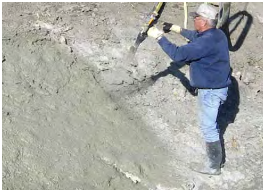
Figure 4. Sprayable ECC applied to irrigation channel repair. Image courtesy of LFL & Associates, 2008.
