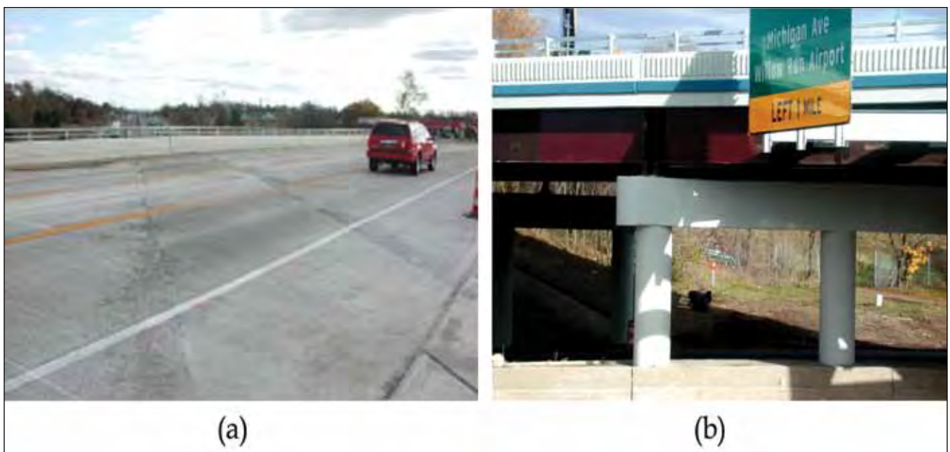
Figure 7. (a) ECC link-slab on (b) Grove Street Bridge in Ypsilanti, MI. Image courtesy of Lepech and Li, 2009.
