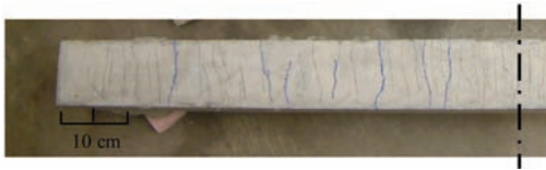
Figure 9. Experimentally observed surface cracking of ECC repair layer. This picture shows a half of ECC repair system. The blue marks indicate the cracks with the width between 40 \mu\text{m} and 60 \mu\text{m} , and the black marks indicate the cracks with the width smaller than 40 \mu\text{m} .
